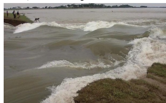
Figure 5.3. Broken embankment in Tahirpur district, Northeast Bangladesh
